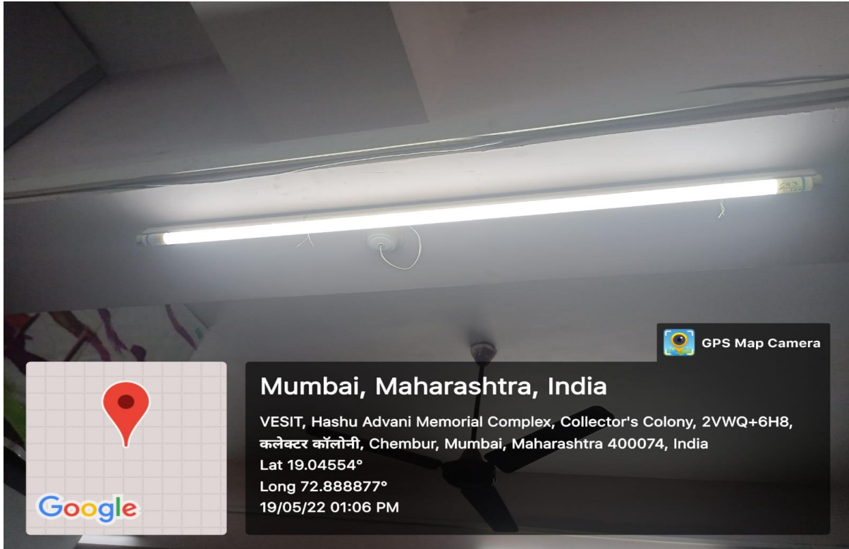
Figure- LED lights installed in corridor
