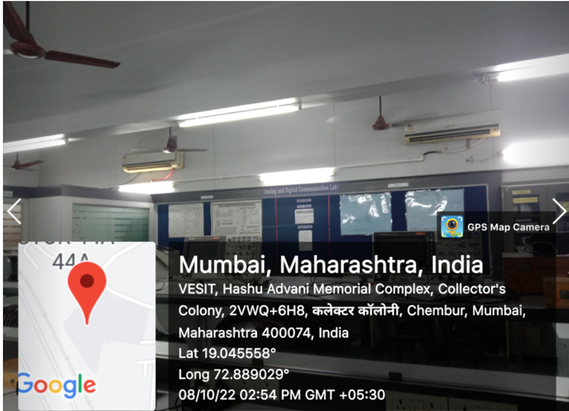
Figure- LED lights installed in laboratories
