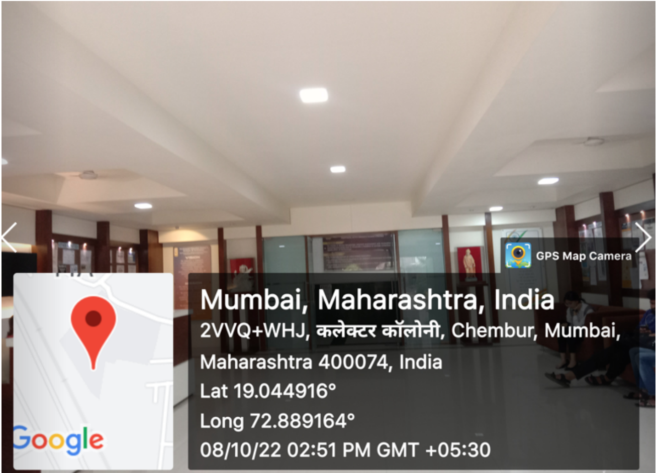
Figure- LED lights installed at entrance
